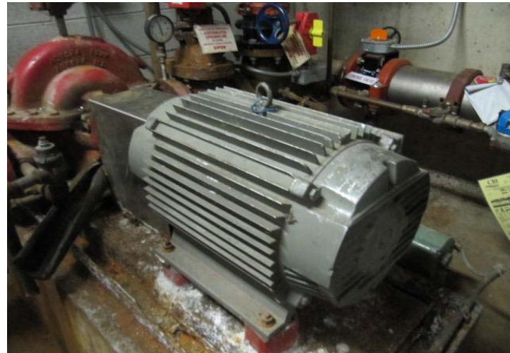
Fire pump, in functional condition at 30 years of age.
