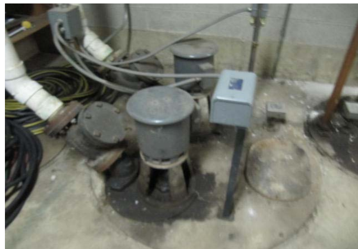
Sump pumps vary in age and condition.
