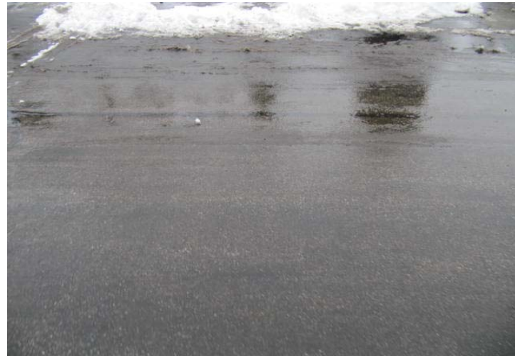
Pavement is smooth and level.
