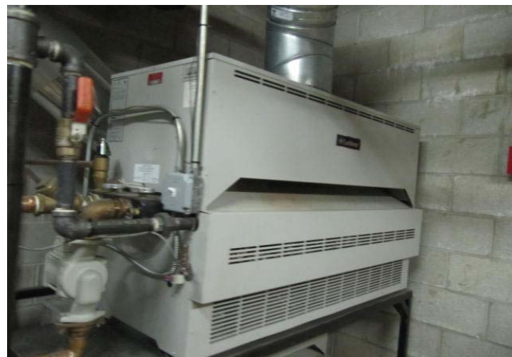
Boilers are in good operational condition.
