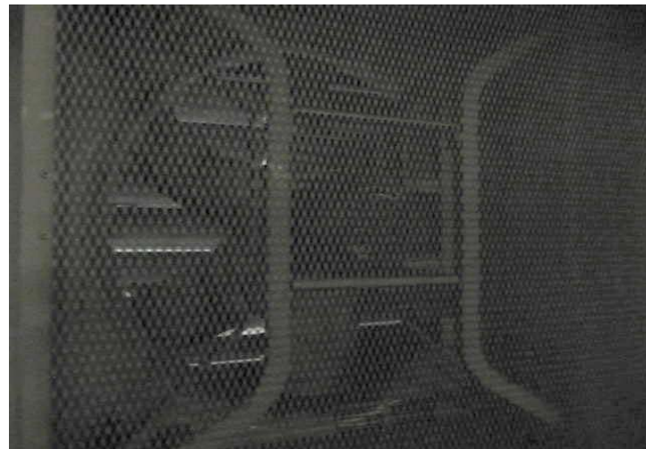
Interior of exhaust fan, with axial blades and motor.
