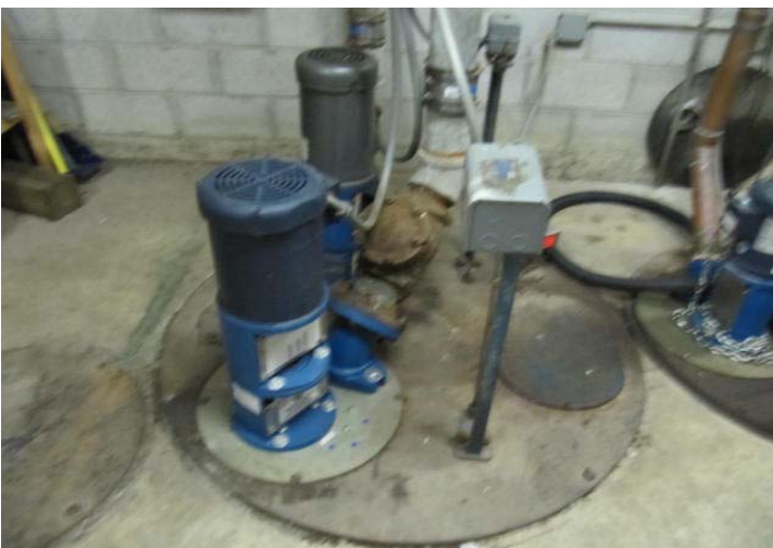
Sump pumps vary in age and condition.
