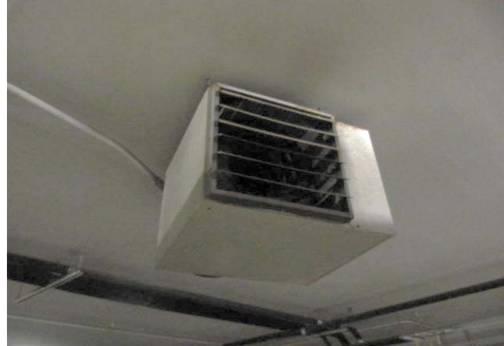
Electric unit heater at parking garage.
