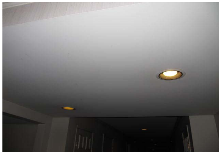
Painted ceiling surface at hallway.
