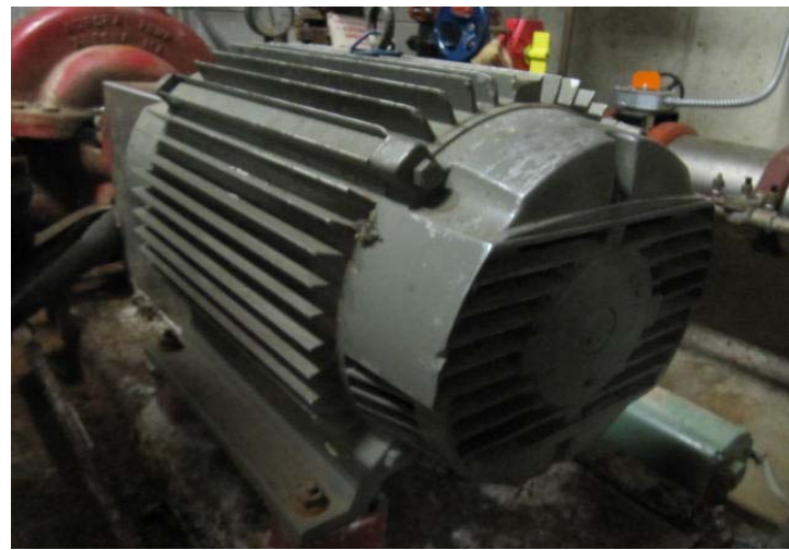
Fire pump, rated for 30-Horespewr.
