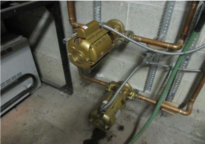
Overview of domestic hot water circulation pump.
