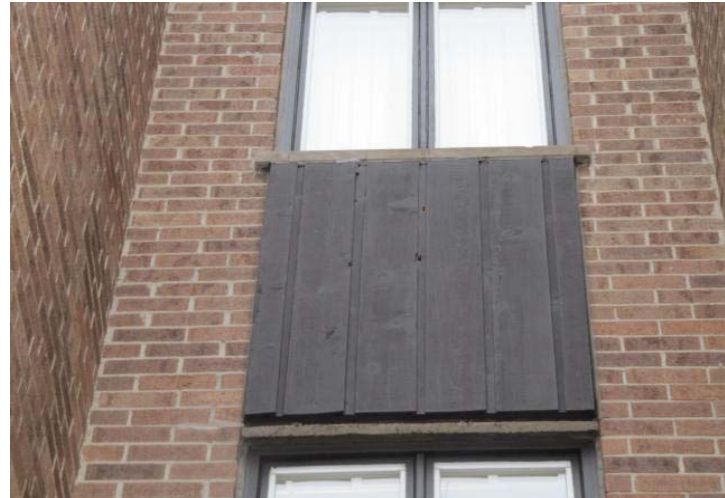
Original wood siding, at 30 years of age.
