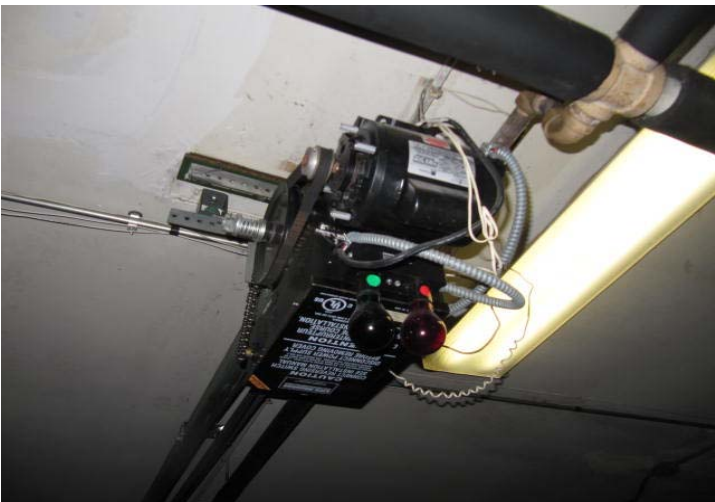
Garage door operator, with red/green lights.
