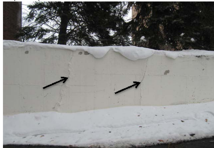
Various cracks at concrete retaining walls.
