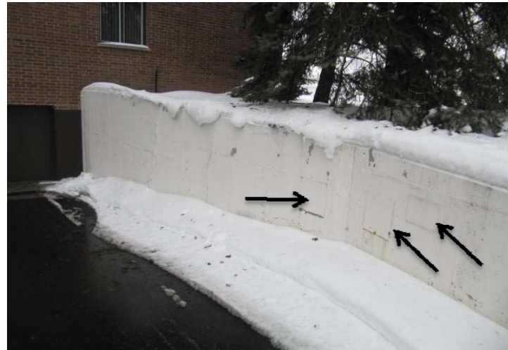
Retaining wall along garage entrance drive, with evidence of past repairs.
