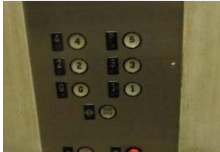
Floor selector buttons at cab interior.
