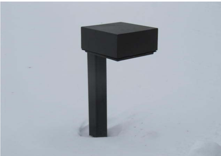
Shorter path light along fire lane.
