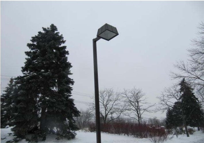
Typical single-fixture light pole at parking lot.
