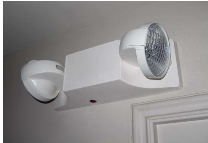
Newer emergency light fixture in good condition.
