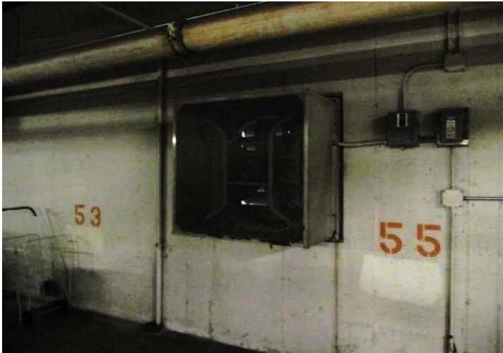
Overview of garage exhaust fan.
