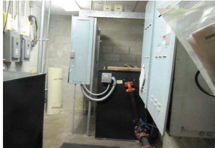
Overview of hydraulic elevator power unit.
