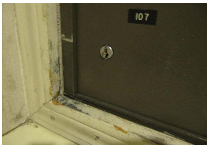
Wood trim at mailbox surround is in poor condition.
