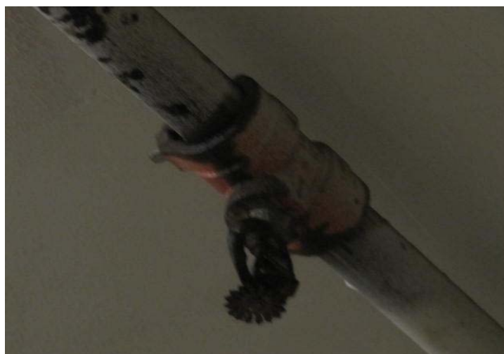
Typical fire sprinkler head.
