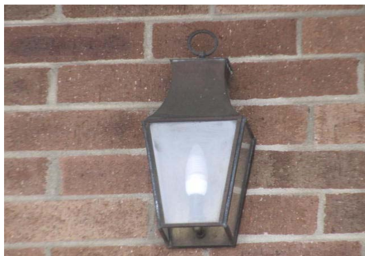
Typical wall sconce at unit balcony.
