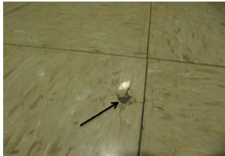
Cracked, damaged vinyl tile at lower level elevator lobby.
