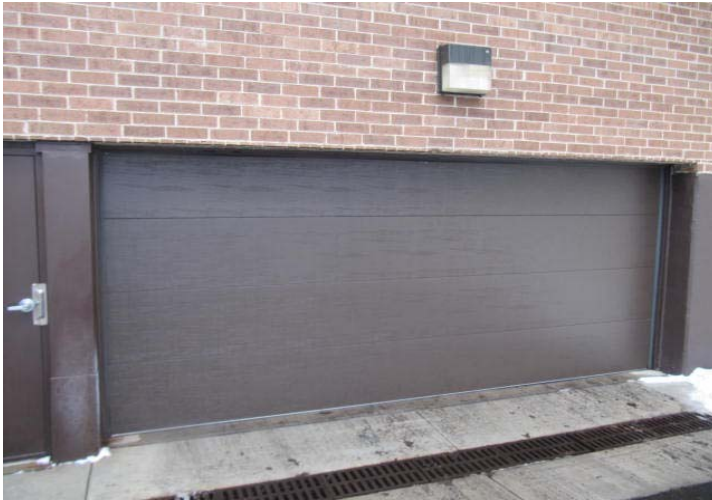
Overview of metal sectional garage door.
