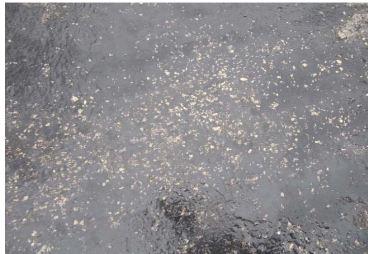
Typical surface condition at fire lane pavement.
