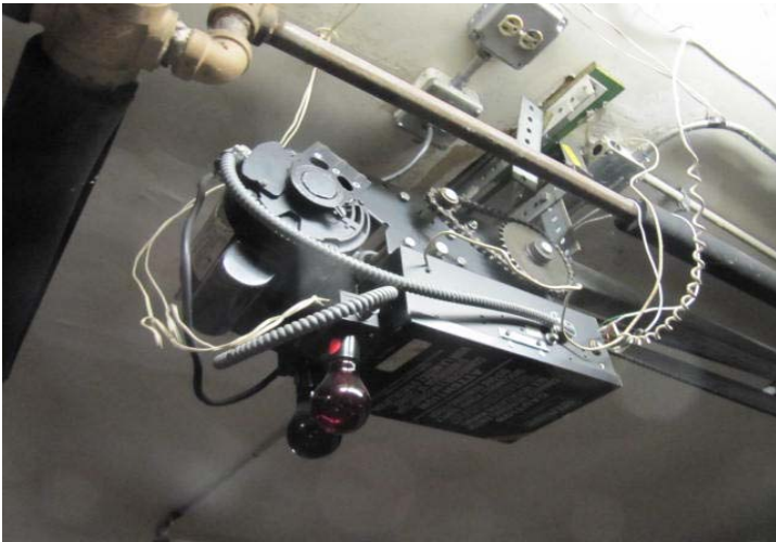
Garage door operator.
