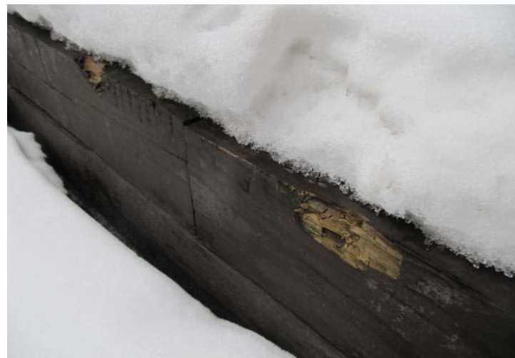
Chipped timber member, with exposed wood.
