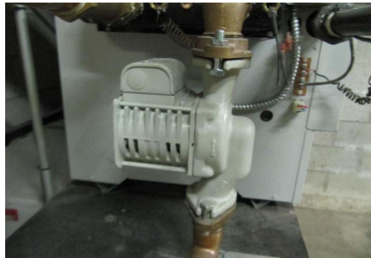
Circulating pump for domestic hot water.
