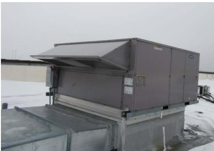
Overview of rooftop heating and cooling unit.
