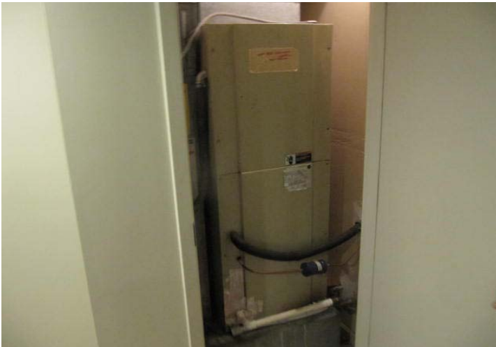
Overview of fan coil unit serving meeting room.
