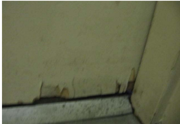
Deteriorating wood door leaf, near grade.
