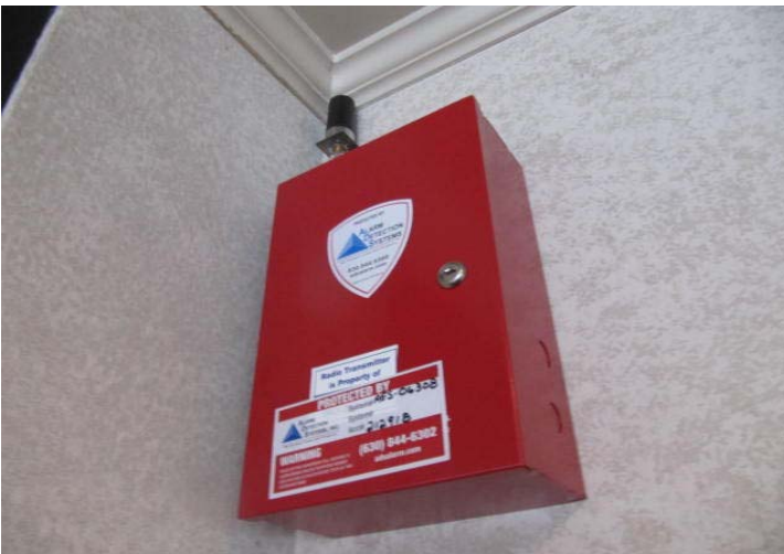
Wireless transmitter for fire control panel.
