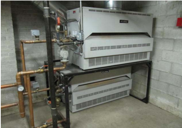
Overview of boilers providing domestic hot water.
