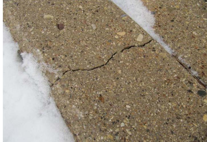
Cracked concrete curb at parking lot.
