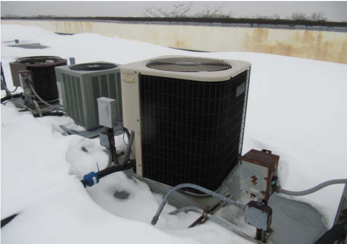
Overview of condensing unit at building rooftop.
