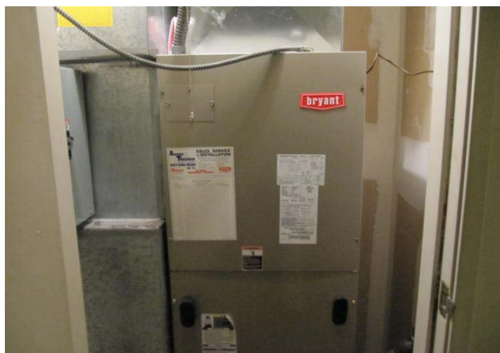
Bryant brand fan coil unit.
