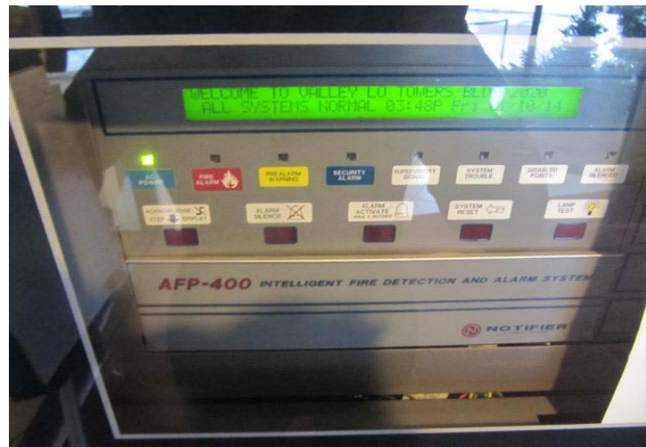
Digital display at fire control panel.
