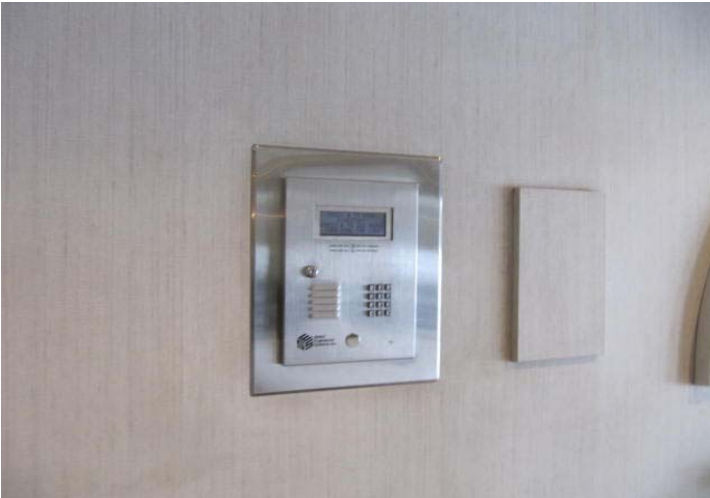
Overview of intercom entry panel.
