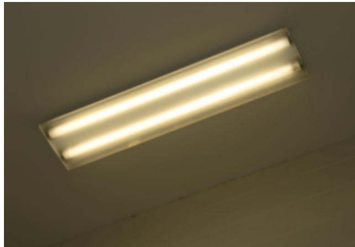
Interior light fixture at interior private stairwell.
