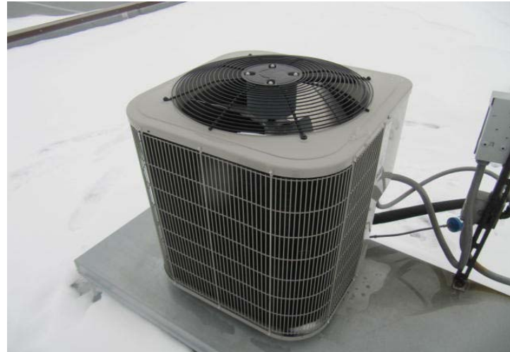
Condensing unit for exercise room.
