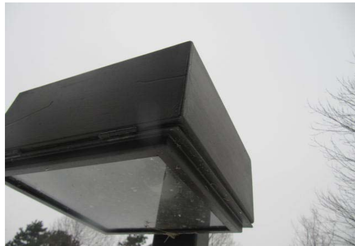
Typical light fixture along fire lane.
