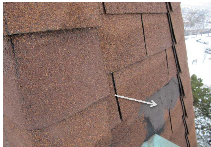
Evidence of past repairs / patching at roof.
