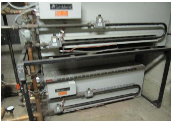
Lochinvar boilers at garage-level mechanical room.
