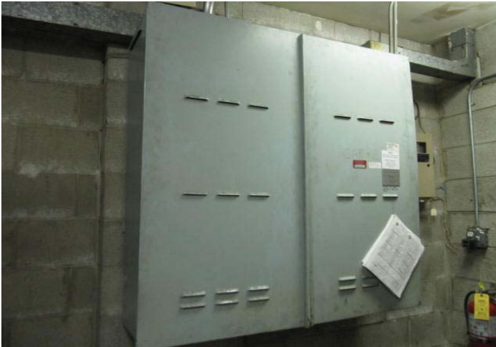
Overview of elevator controller.
