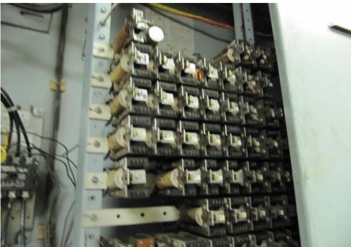
Original elevator controls, at 30 years of age.
