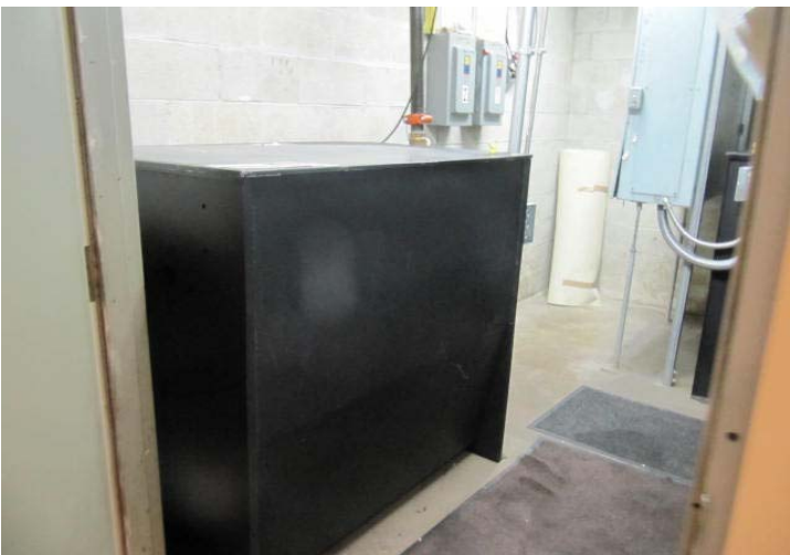
Hydraulic power unit, replaced in 2005 - 2006.
