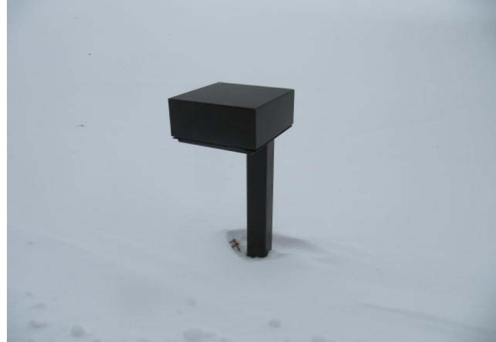
Typical light fixture along fire lane.
