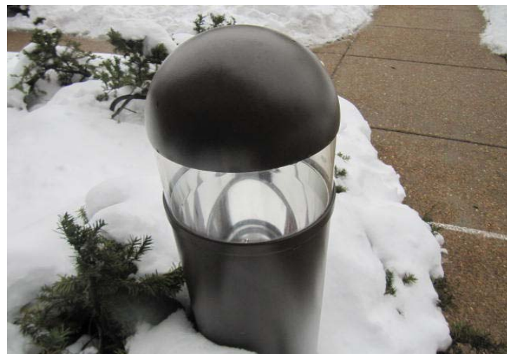
Newer bollard light fixture, in very good condition.
