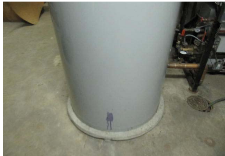
Storage tank with 200-Gallon capacity.
