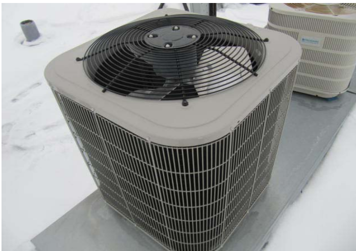
Condensing unit, replaced in 2011.
