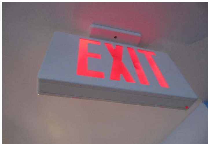
Ceiling mounted double-sided emergency exit sign.
