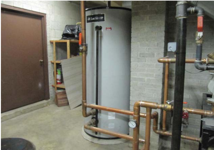
Overview of domestic hot water storage tank.
