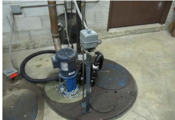
Sump pump station with controls.
