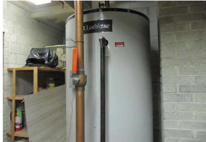
Lochinvar hot water storage tank.
