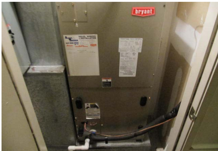
Overview of fan coil unit serving exercise room.
