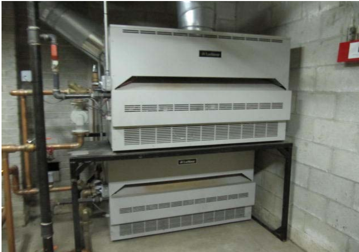
Overview of boilers providing domestic hot water.
