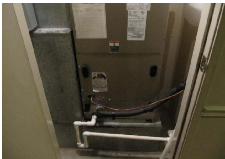
Fan coil unit located at hallway closet.
