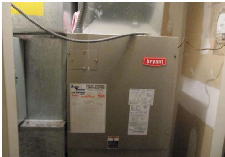
Fan coil unit, replaced in 2011.
