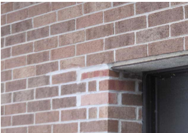
Evidence of past repointing at masonry mortar joints.
