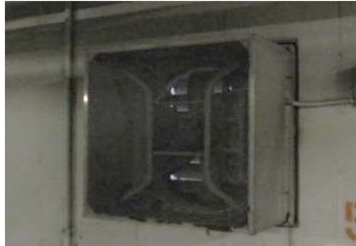
Typical sidewall garage exhaust fan.
