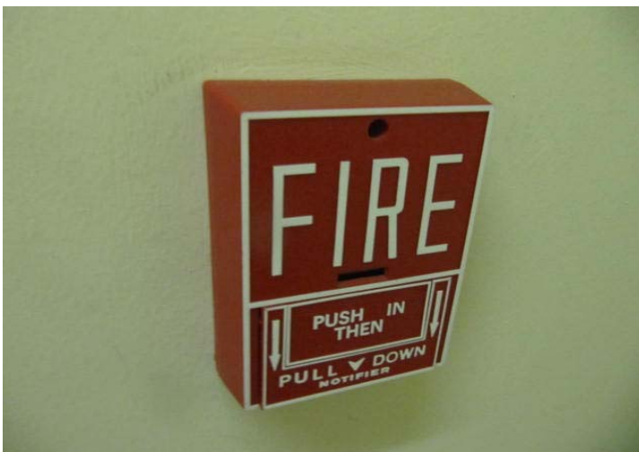
Emergency manual pull station.
