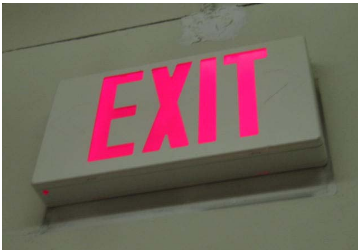
Wall mounted emergency exit sign.
