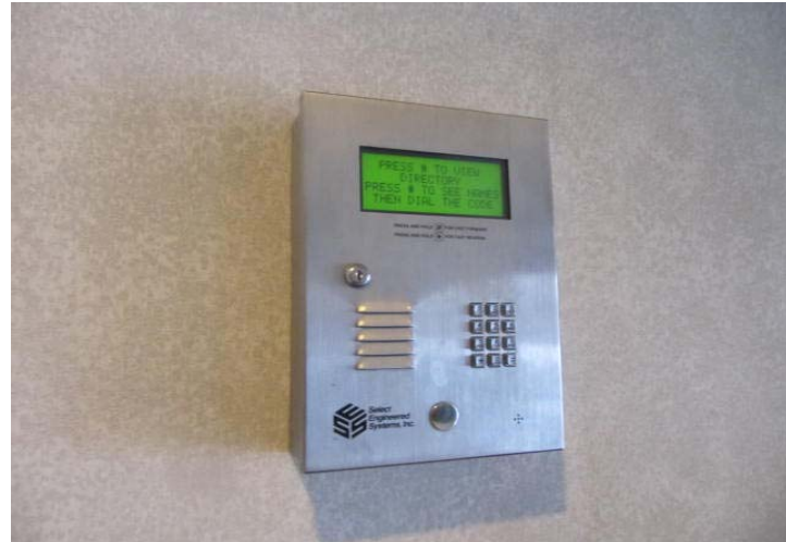
Overview of intercom entry panel.
