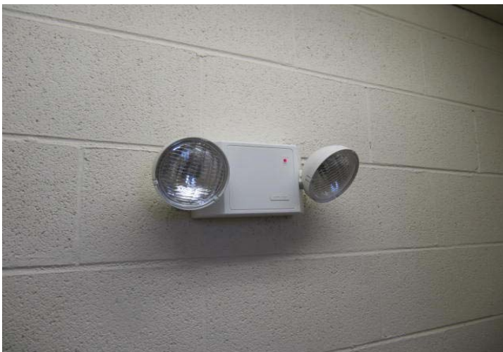
Newer emergency light fixture in good condition.
