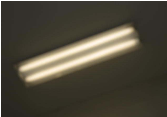
Interior light fixture at interior private stairwell.
