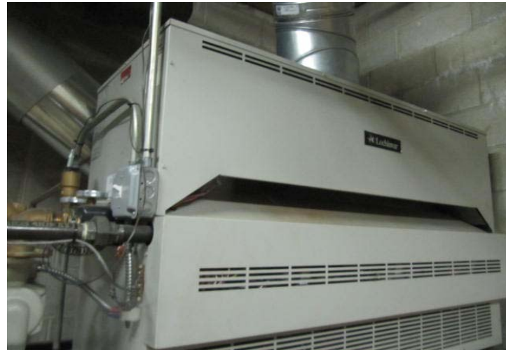
Domestic hot water boilers, at 9 years of age.
