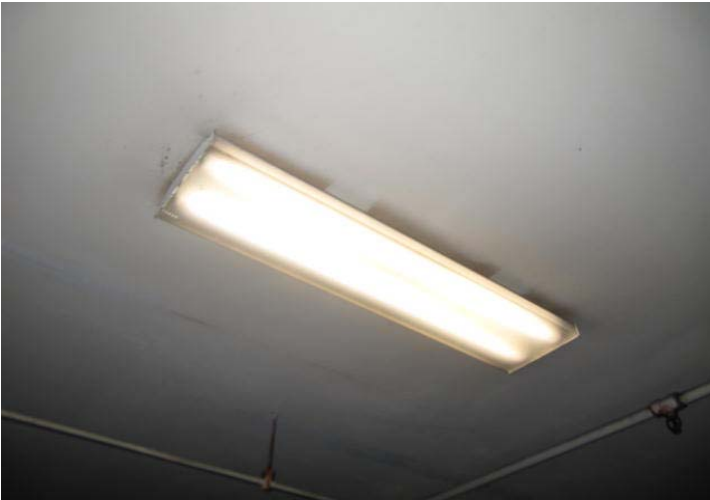
Typical fluorescent light fixture at parking garage.
