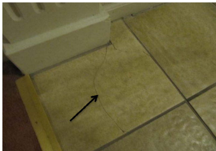
Isolated condition of cracked tile at lobby area.
