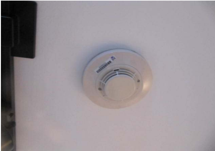
Ceiling mounted smoke detector.
