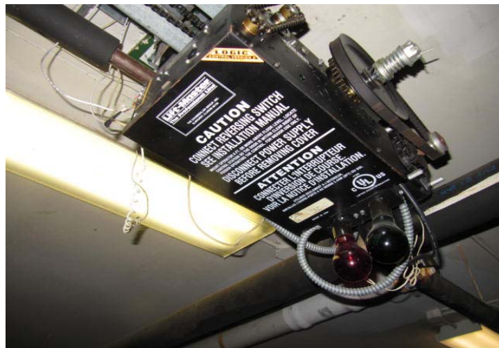
Garage door operator, with red/green lights.
