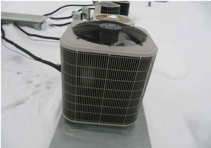
Overview of condensing unit at building rooftop.
