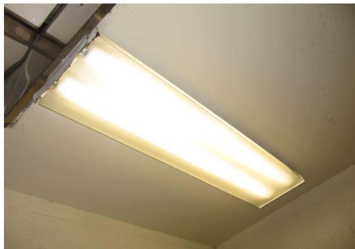
Light fixture at stairwell connected to hallway.
