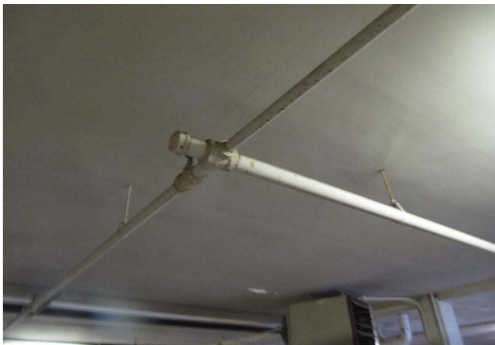
Overview of piping for fire suppression system.
