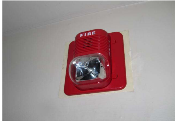
Wall mounted horn / strobe.
