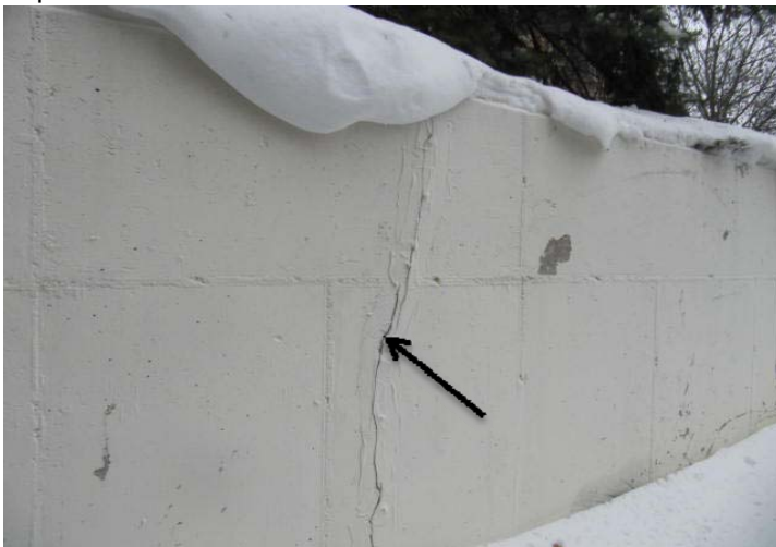
Crack at concrete retaining walls.
