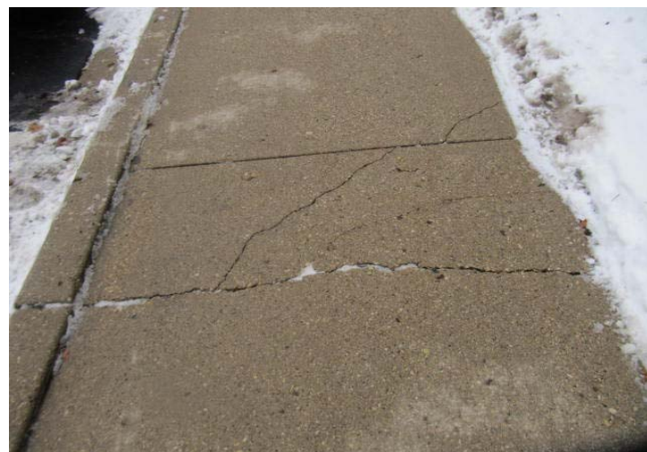
Cracked concrete flatwork at sidewalk.
