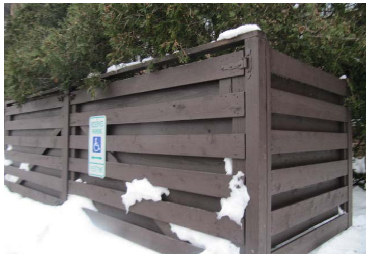
Painted transformer enclosure.
