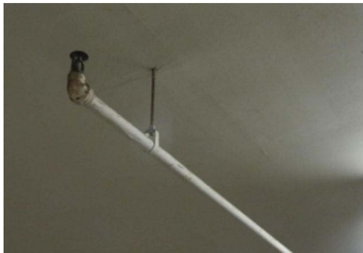
Sprinkler system piping and sprinkler head.
