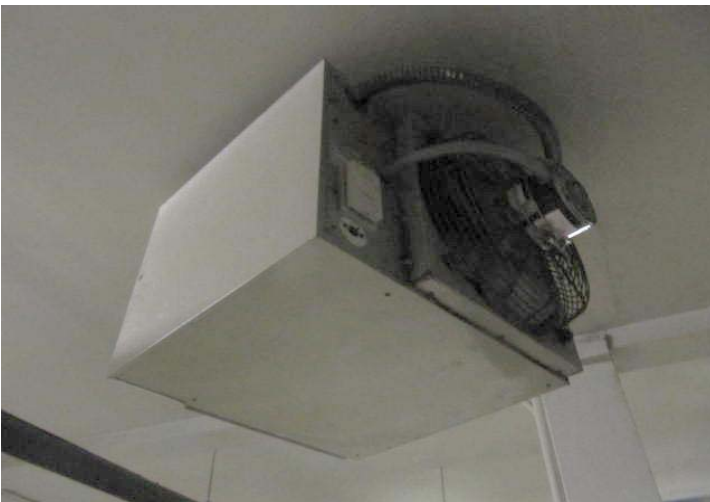
Electric unit heater at parking garage.
