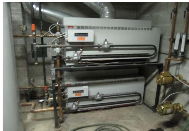
Boilers are in good operational condition.
