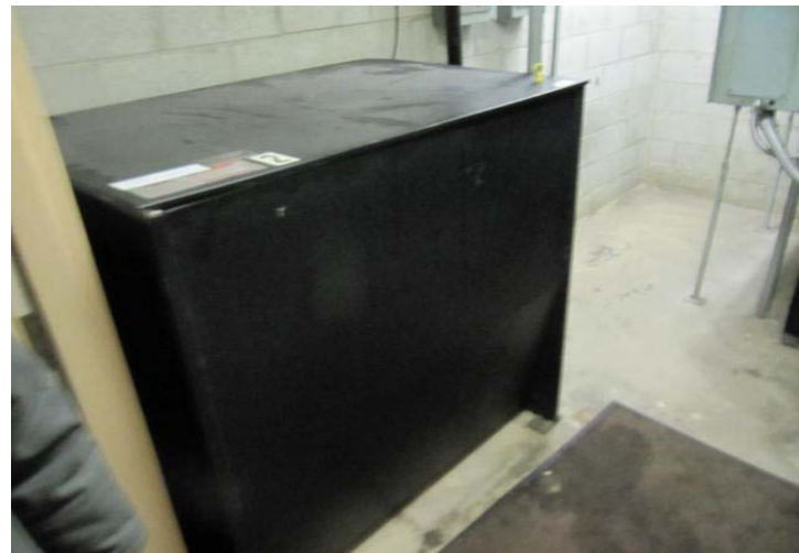
Hydraulic power unit, replaced in 2005 - 2006.
