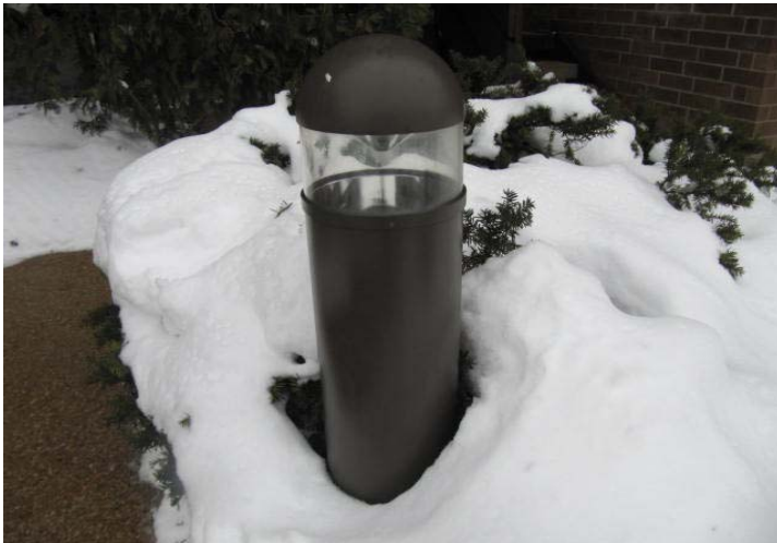
Overview of bollard light fixture.
