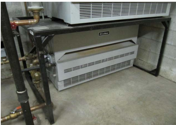
Lochinvar boilers at garage-level mechanical room.
