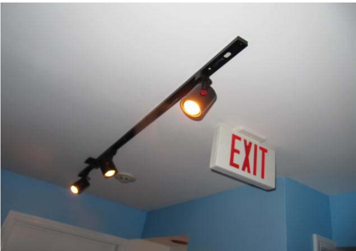
Track light fixture at Exercise Room.
