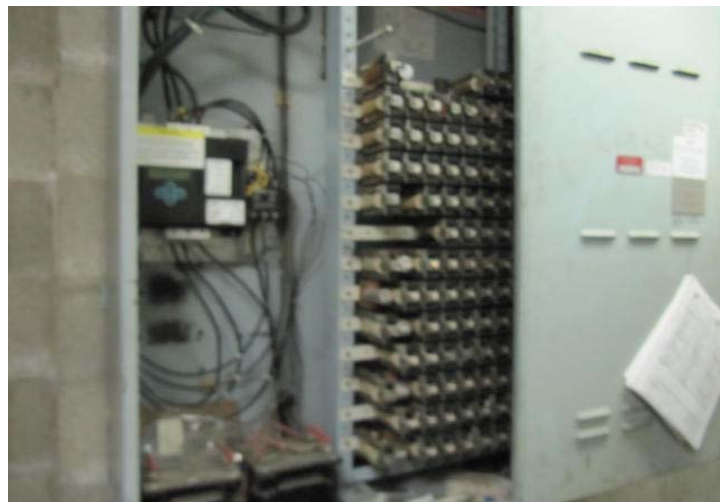
Relay logic circuits at elevator control panel.
