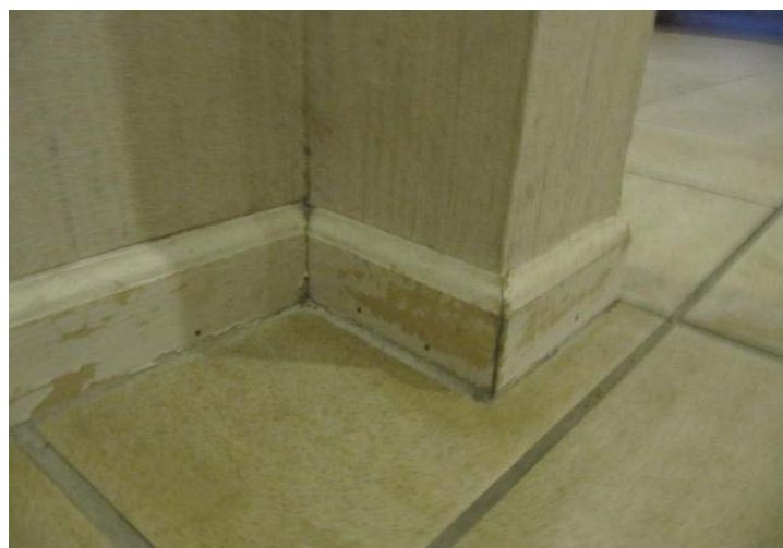
Worn paint finishes at base trim at lobby.
