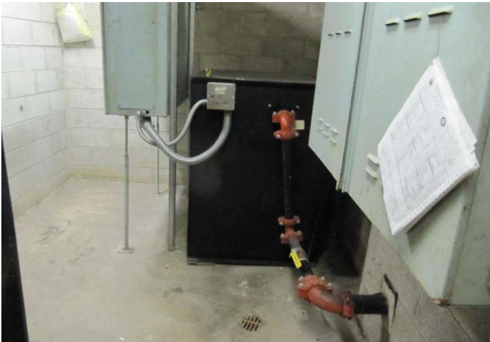
Overview of hydraulic elevator power unit.
