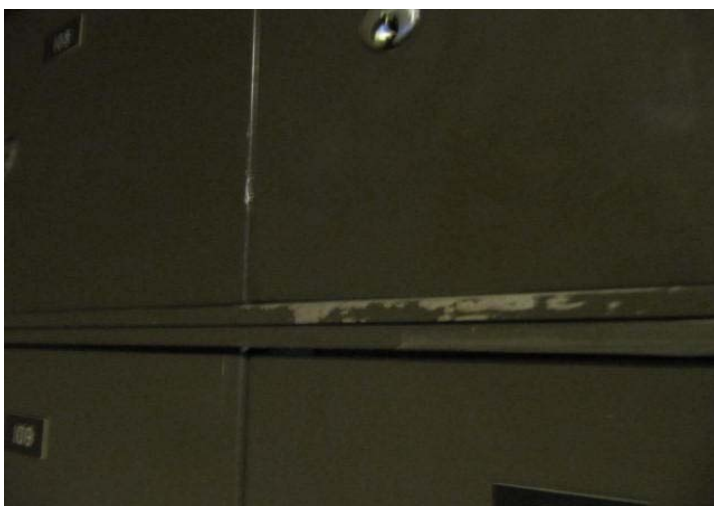
Worn finishes at aluminum mailboxes.
