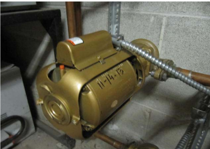
Pump motor, replaced in 2013.
