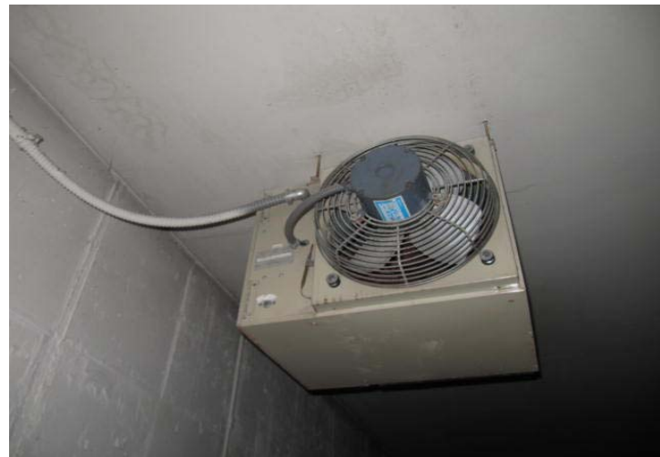
Original unit heater, at 30 years of age.
