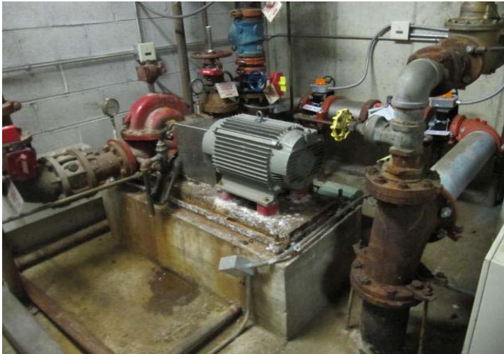
Overview of fire pump.
