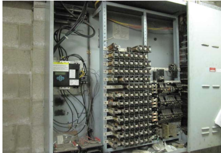
Elevator controller at garage-level equipment room.
