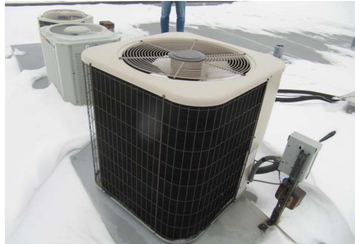
Condensing unit for meeting room.
