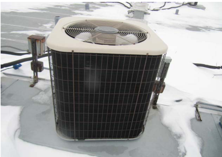
Condensing unit at building rooftop.
