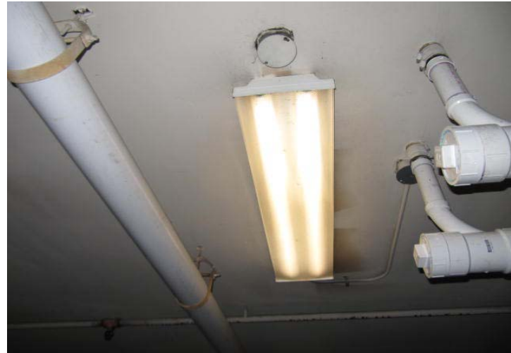
Typical fluorescent light fixture at parking garage.
