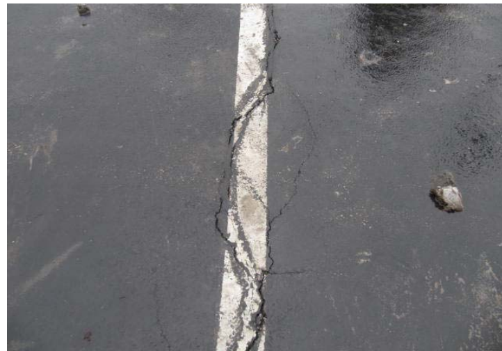
Cracks at asphalt pavement.
