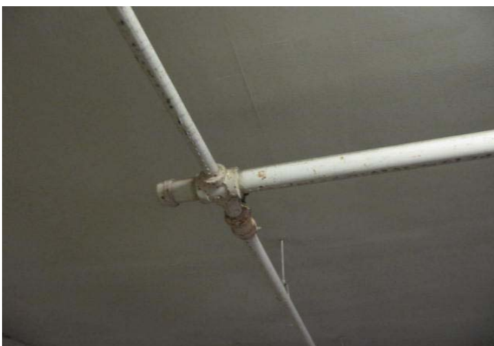
T-section at fire suppression system piping.
