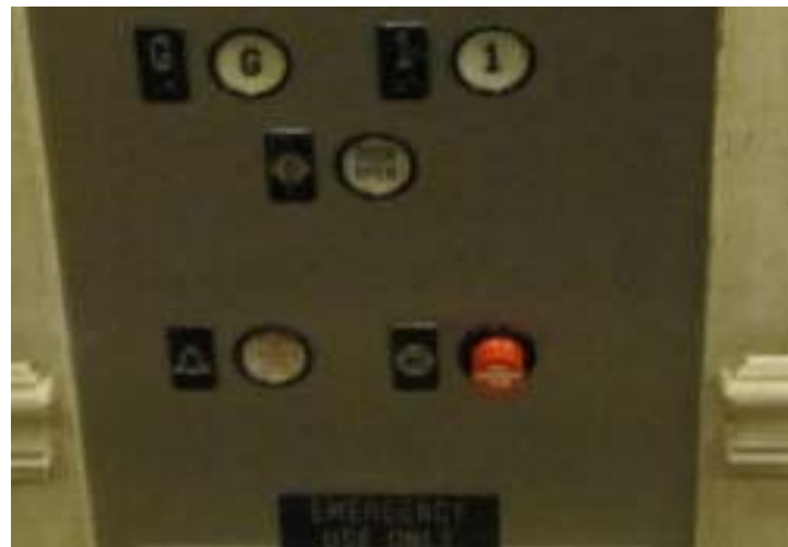
Fixtures at floor selector panel at cab interior.
