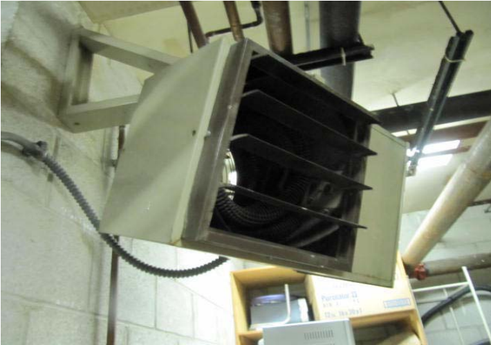
Electric unit heater at mechanical room.
