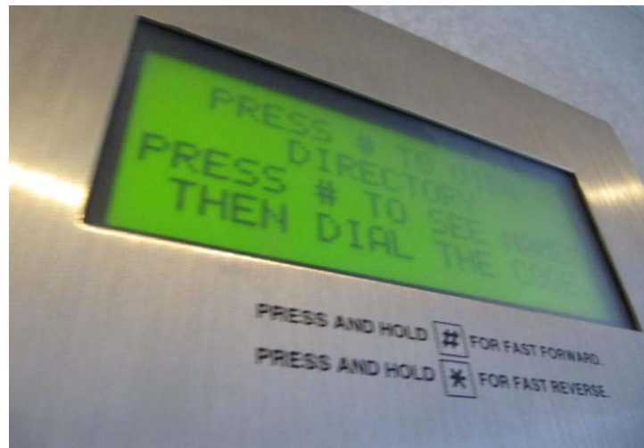
Digital display at intercom entry panel.
