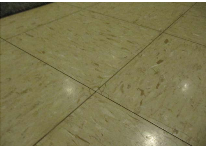
Hairline cracks at vinyl tile at lower level elevator lobby.
