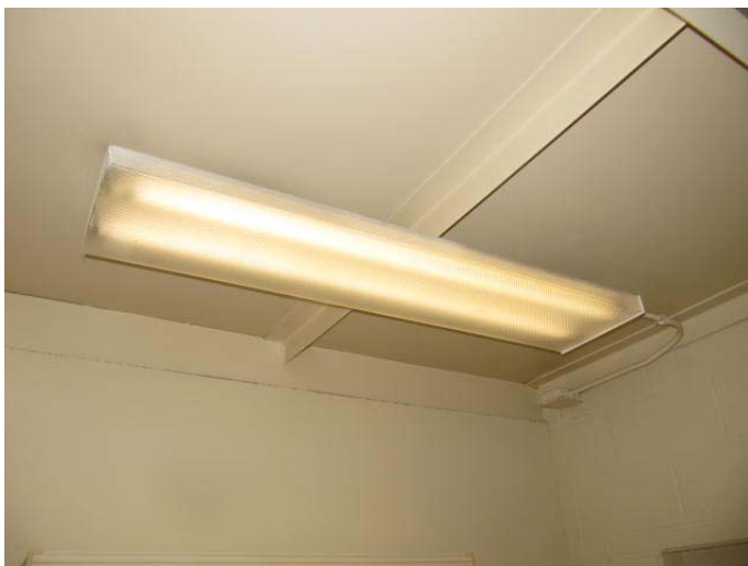
Interior light fixture at stairwell.
