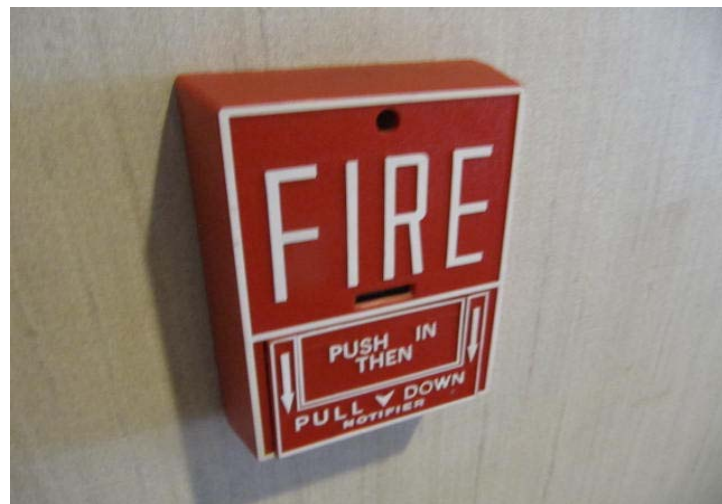
Emergency manual pull station.
