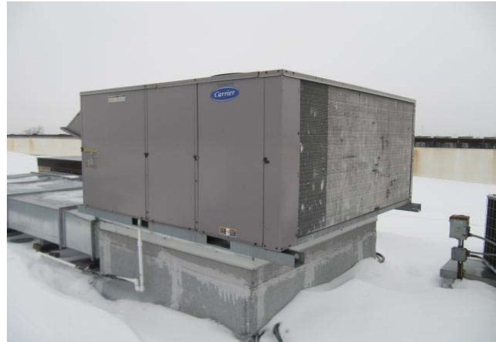
Carrier brand rooftop heating and cooling unit.
