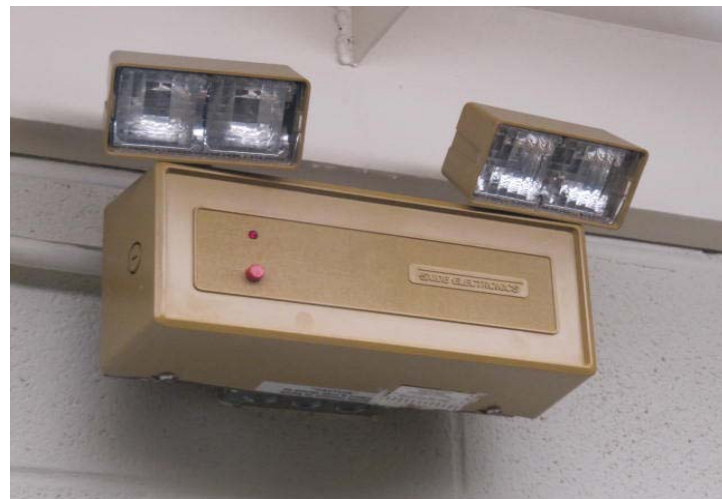
Older emergency light fixture, in functional condition.
