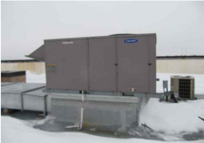
Overview of rooftop heating and cooling unit.
