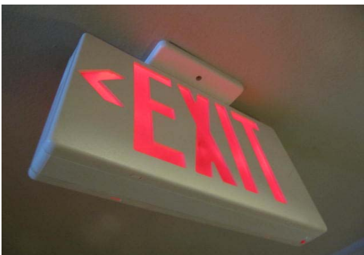
Ceiling mounted double-sided emergency exit sign.
