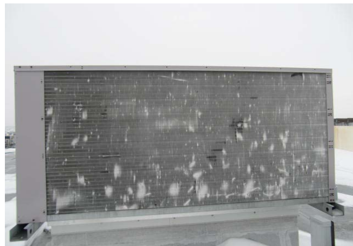
Side view of rooftop heating and cooling unit.
