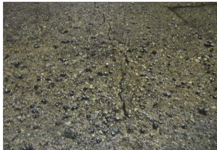
Pitted concrete near garage entrance.
