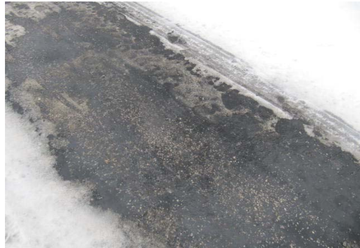
Typical surface condition at fire lane pavement.
