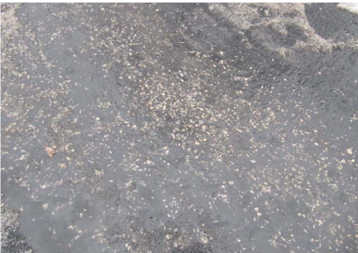
Typical surface condition at fire lane pavement.
