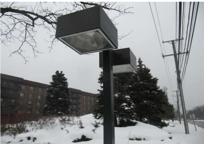
Duplex fixture near property entrance.
