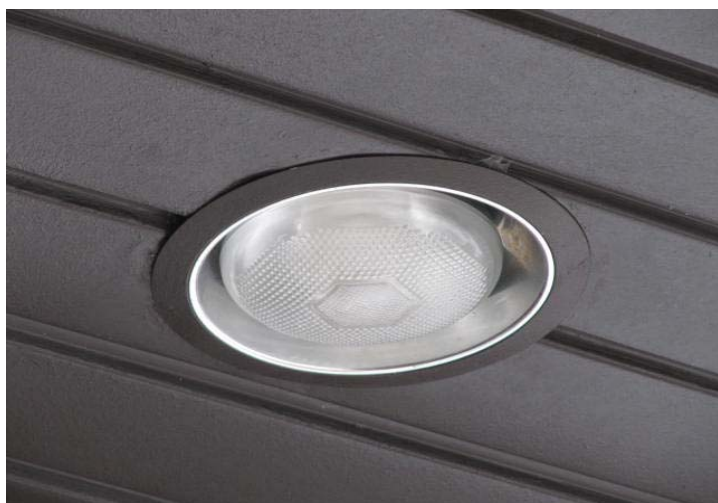
Recessed can fixture at entry soffit.
