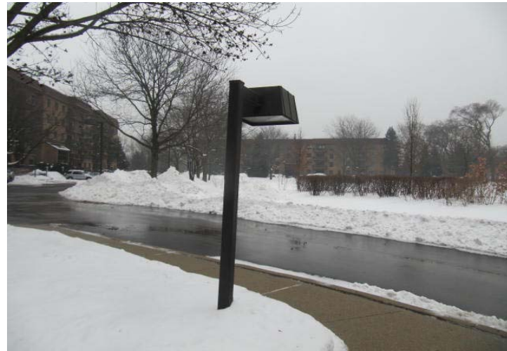
Typical single-fixture light pole at parking lot.
