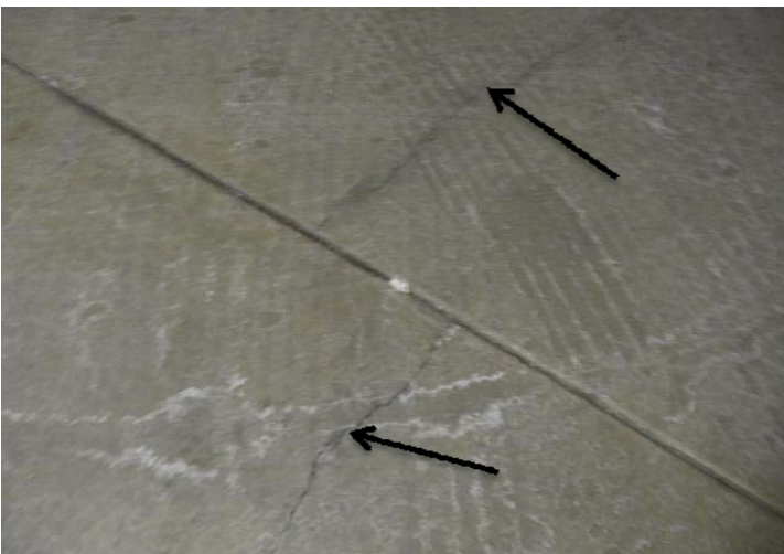
Hairline cracks at concrete garage floor.
