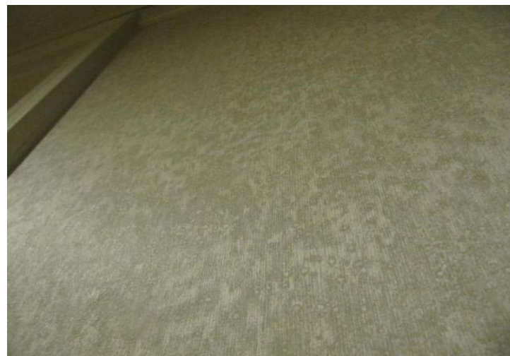
Typical surface condition at wall coverings at lobby.
