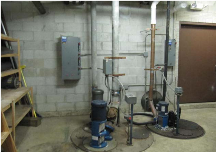
Overview of sump pump stations at mechanical room.
