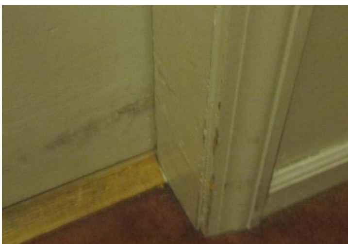
Worn paint finishes at trim; Markings at painted door.
