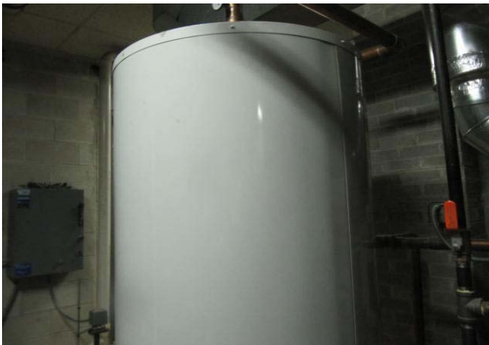
Hot water storage tank, in good condition.
