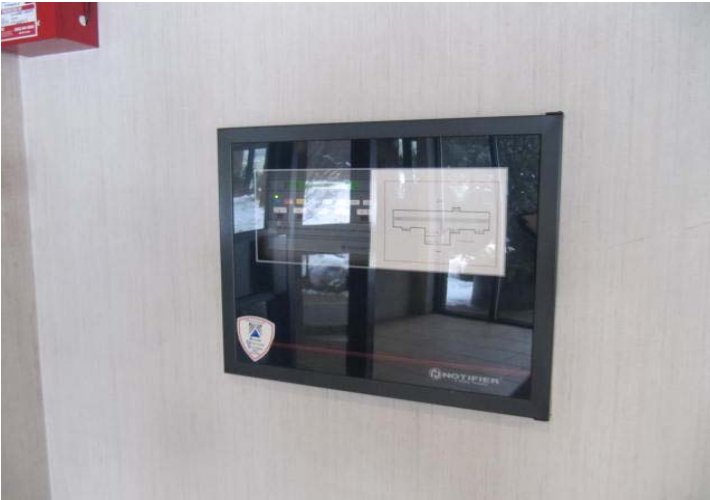
Overview of fire control panel at lobby.
