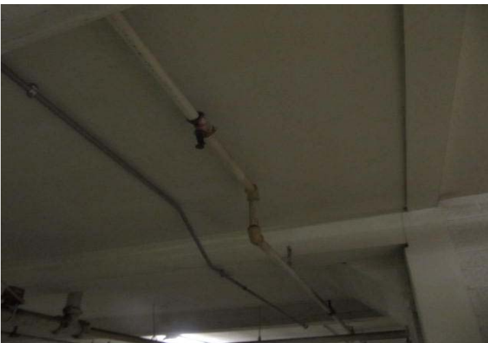
Painted ceiling surfaces at parking garage.
