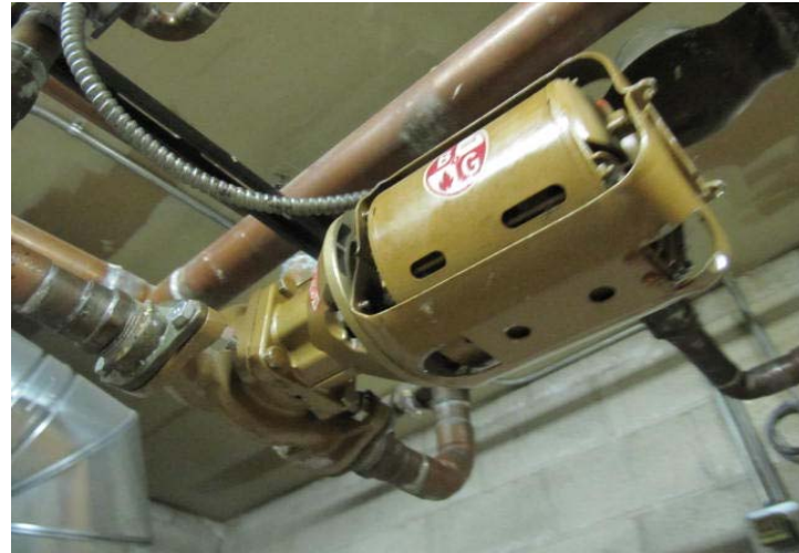
Circulating pump for domestic hot water.
