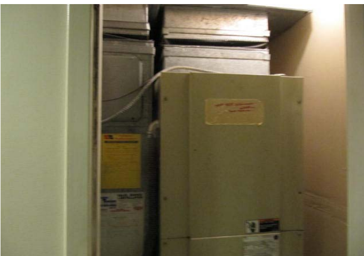
Fan coil unit located at hallway closet near meeting room.
