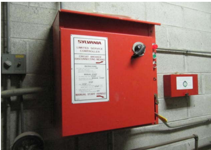
Sylvania Limited Service Controller with manual start.
