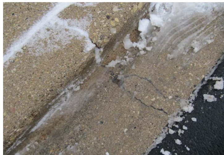
Cracked concrete curb and gutter at parking lot.
