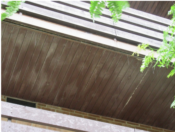
Evidence of water infiltration
