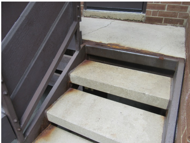
Concrete cracks and rust
