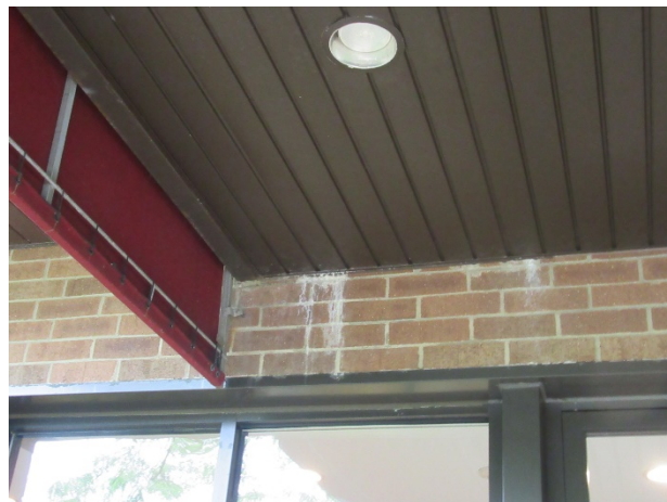
Evidence of water infiltration between canopy and building
