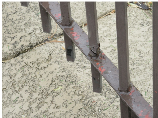
Finish deterioration and rust
