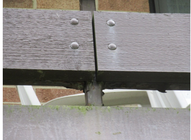
Finish deterioration at metal support
