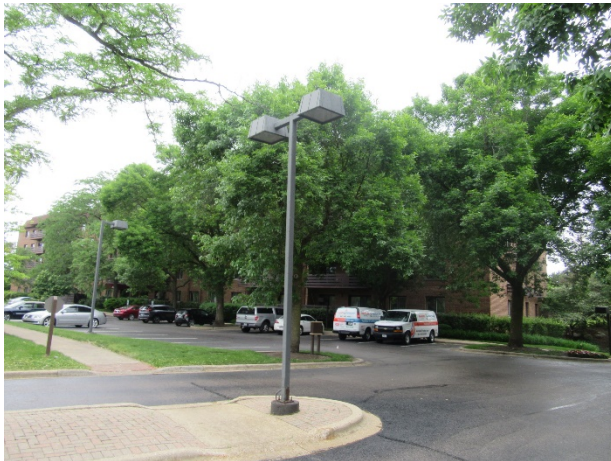
Light pole and fixtures
