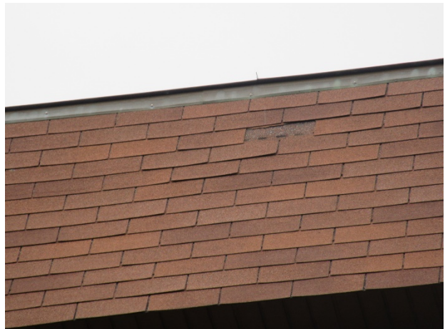
Missing and loose shingles
