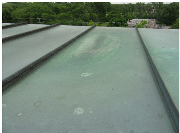
Evidence of water accumulation at metal coping
