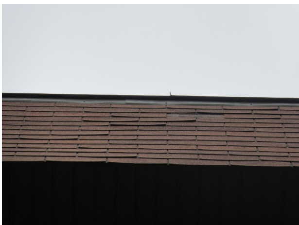
Missing and loose shingles
