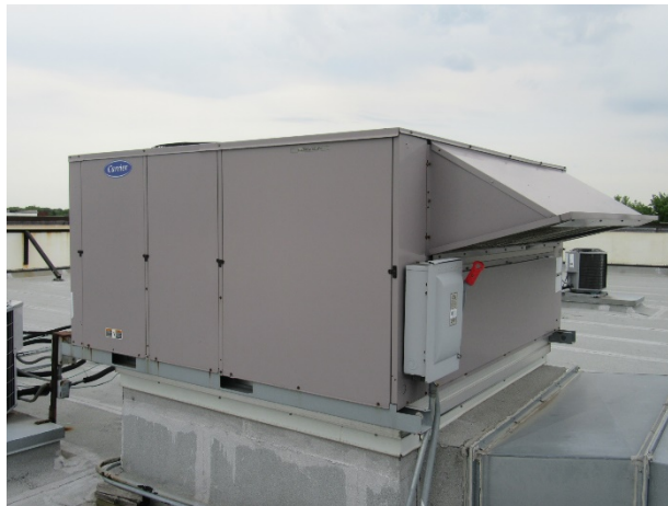
Rooftop heating and cooling unit
