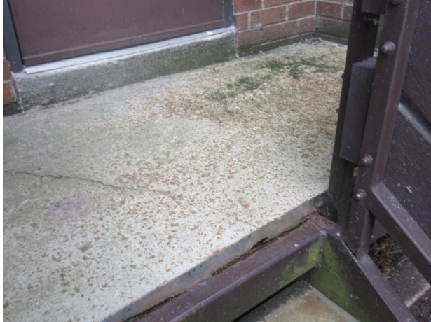
Concrete crack and spall
