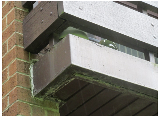
Rust and evidence of water infiltration
