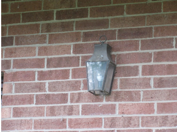
Typical light fixture
