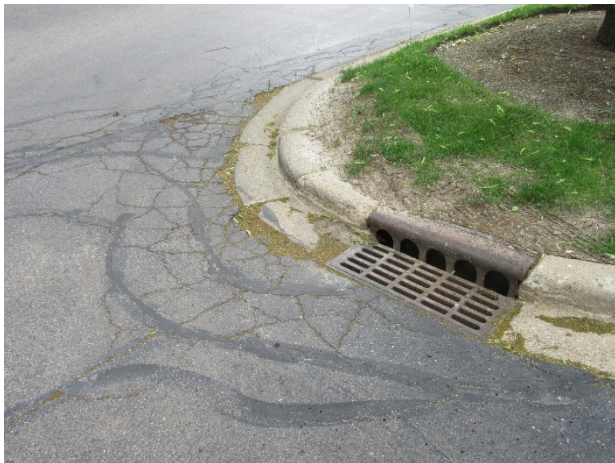
Alligator cracks near catch basin
