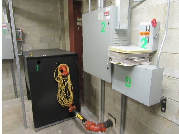
Power unit and controls
