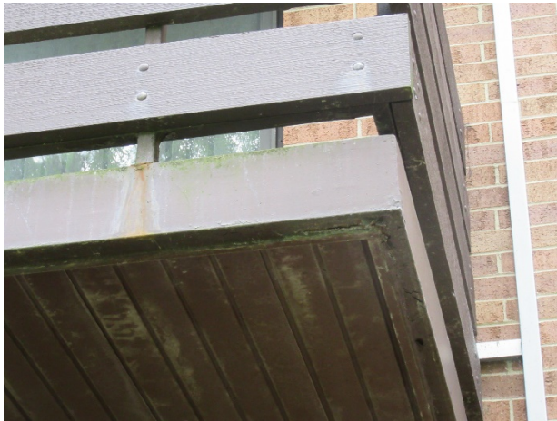
Rust and evidence of water infiltration
