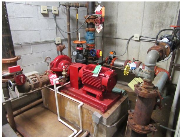
Fire suppression system pump
