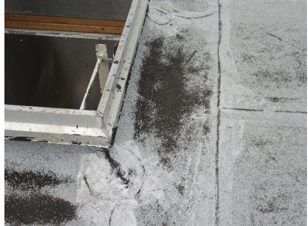
Granular loss near roof access
