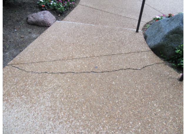
Crack at exposed aggregate sidewalk
