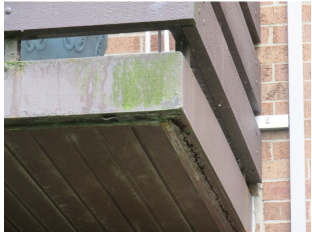
Rust and evidence of water infiltration
