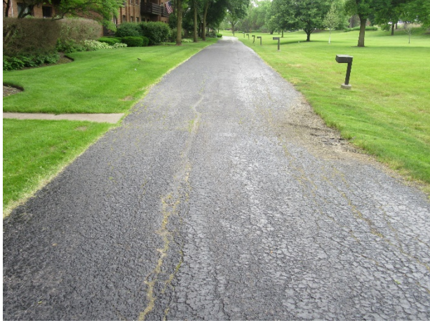
Fire lane overview (note significant cracking)
