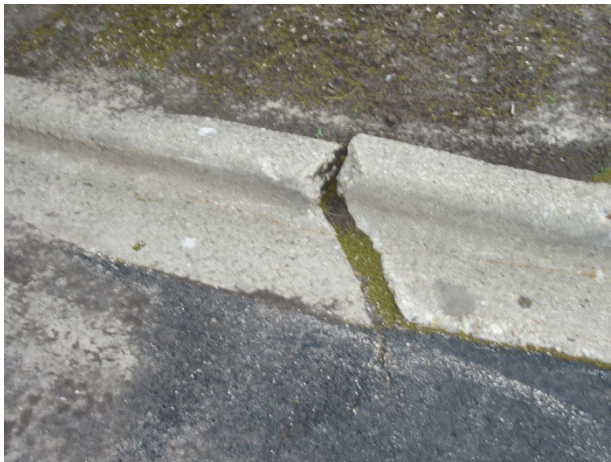
Curb crack and settlement
