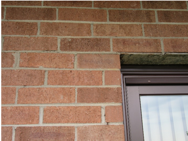
Mortar crack at lintel
