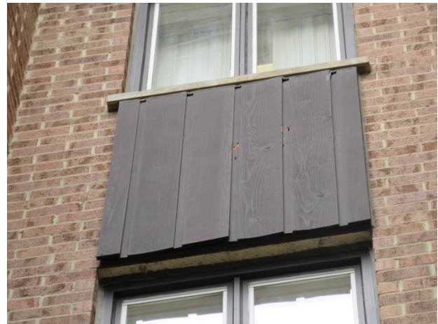
Deflection and damage
