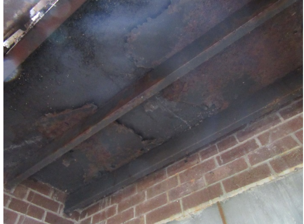
Finish deterioration and rust
