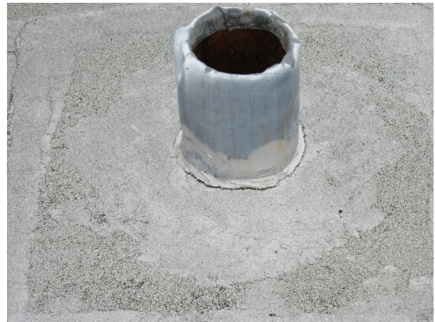
Gap at penetration sealant
