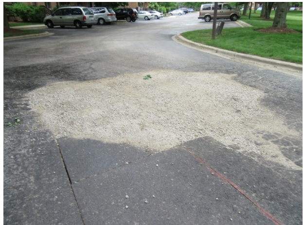
Pavement deterioration near the east garage of the 2000 building
