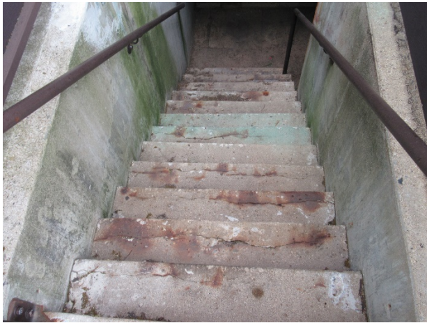
Cracks and rust from reinforcement bars
