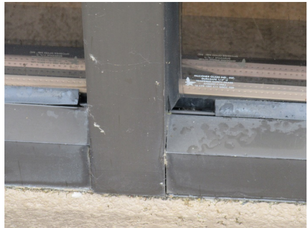
Missing sealant at atrium windows
