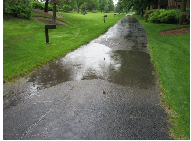
Water accumulation at west end of fire lane
