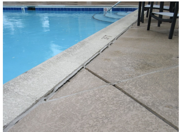
Settlement, sealant adhesion failure and potential trip hazard
