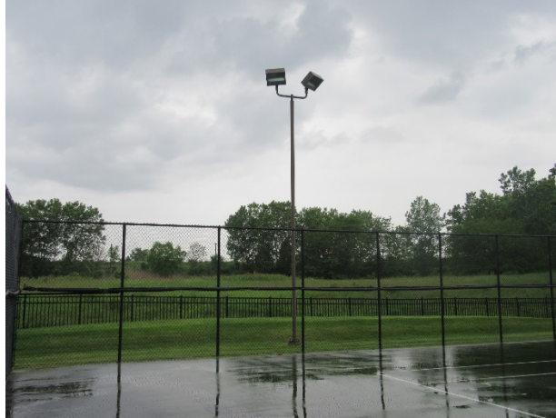
Light pole and fixtures
