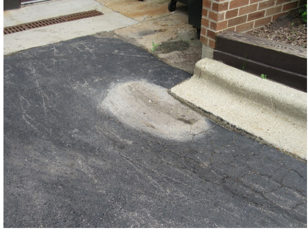
Settlement near west garage of the 2020 building
