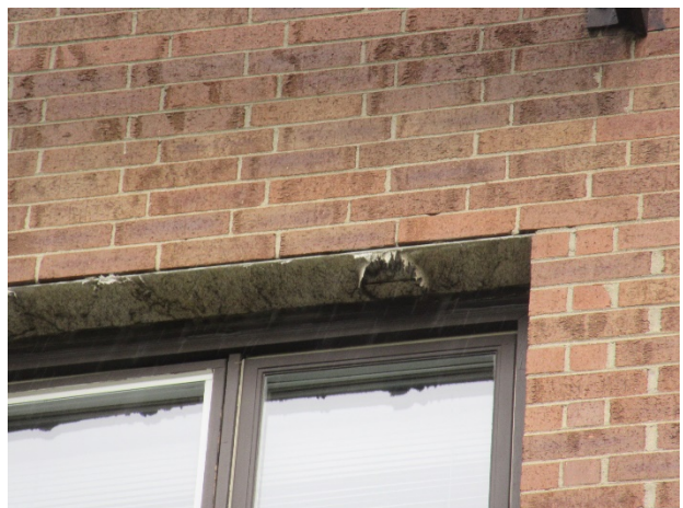
Finish deterioration at lintel
