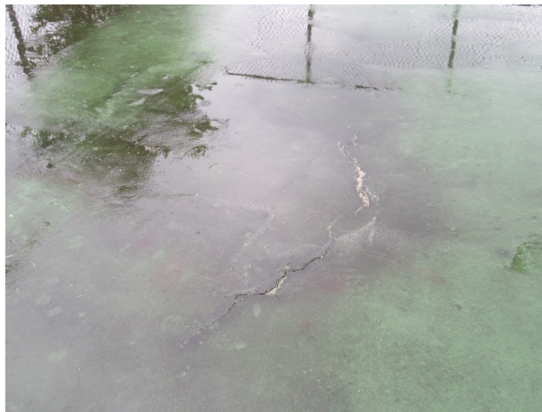
Discoloration and court crack
