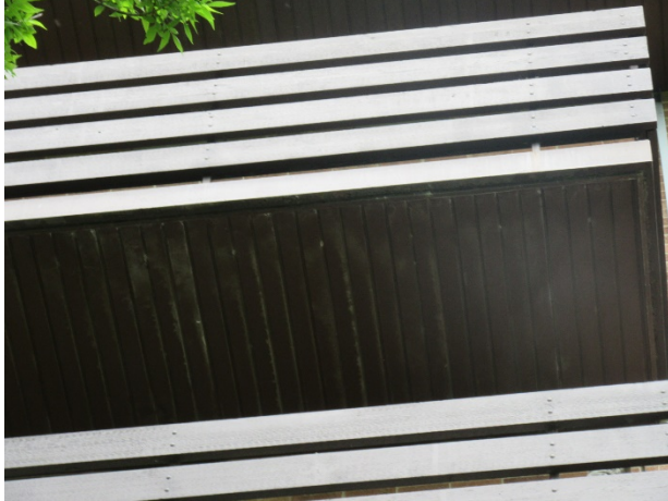
Evidence of water infiltration
