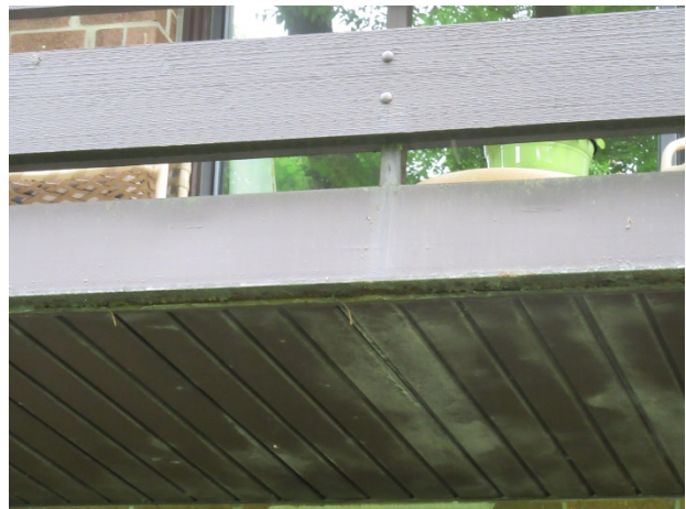
Evidence of water infiltration
