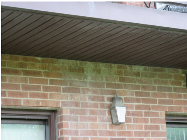
Evidence of water infiltration between balcony and wall
