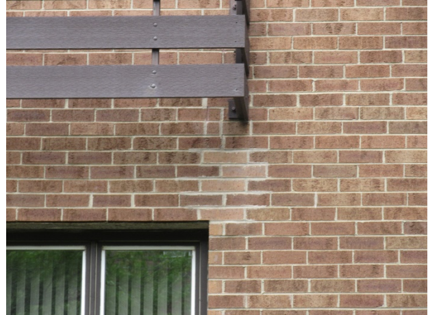
Evidence of prior repairs
