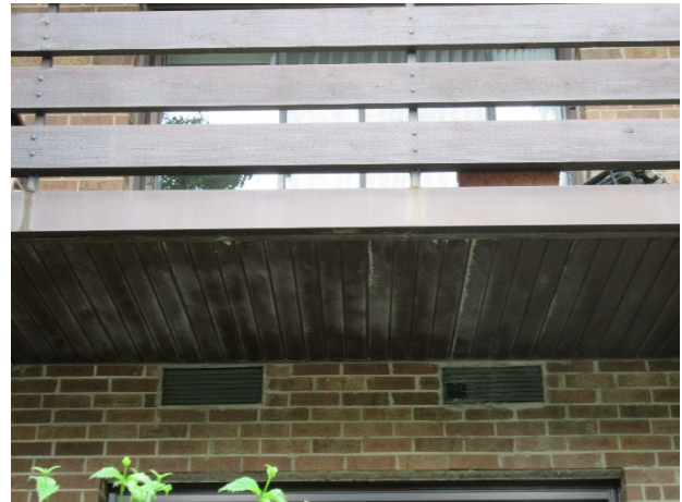
Evidence of water infiltration
