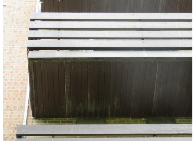
Evidence of water infiltration
