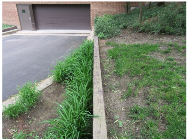
Slight wall lean
