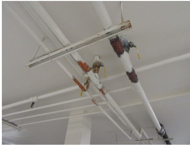
Domestic water pipes
