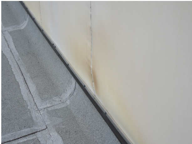
Membrane deflection at parapet wall
