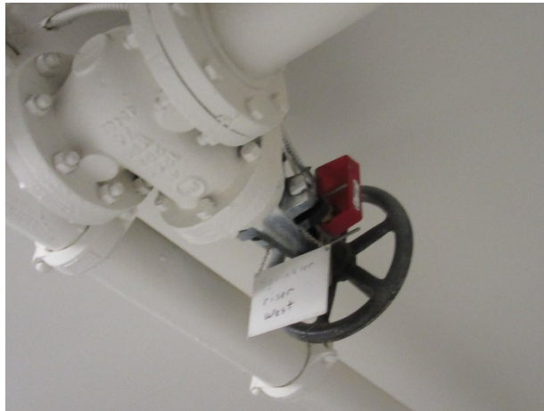
Large diameter valve
