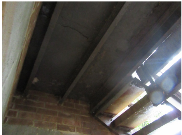
Finish deterioration and rust
